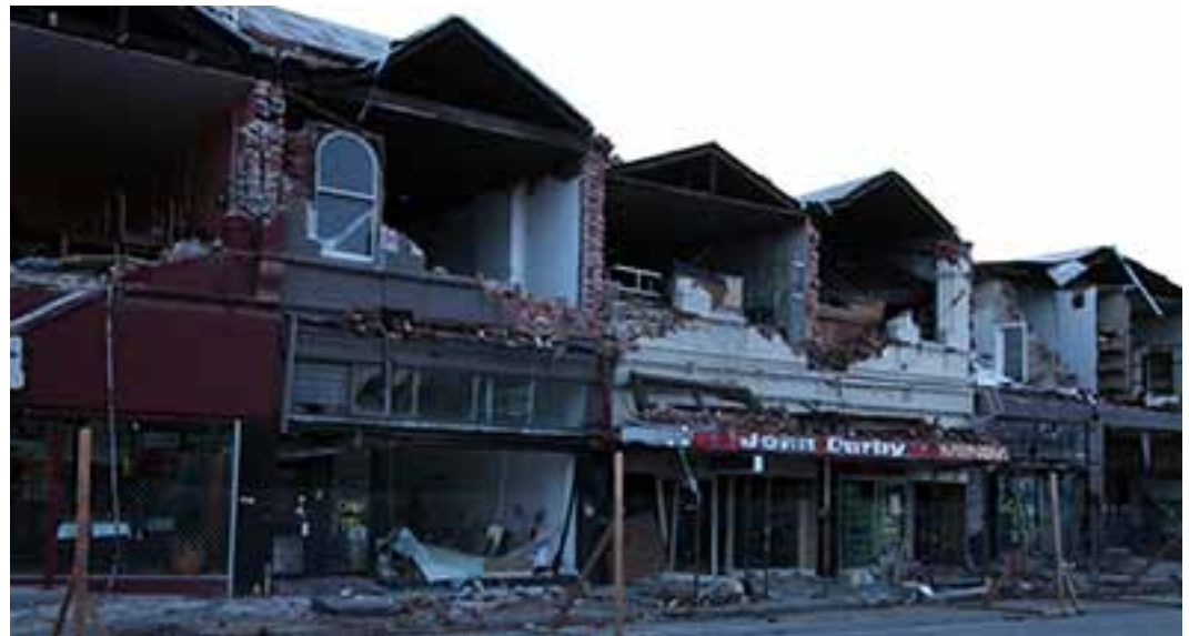
During the February earthquake two-story masonry structures suffered complete facade damage in the Christchurch historical district.
