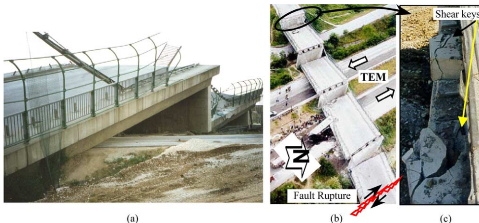
Fig. 9. Arifiye Overpass traversed by surface fault rupture: (a) side view; (b) aerial view [13]; (c) damaged shear keys in the southern bridge abutment.
