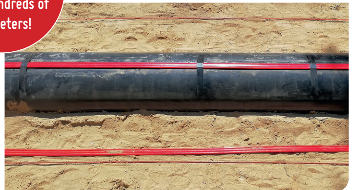
Application of 3DSensor along a gas pipeline
